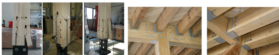
Fig. 7: Examples of connection failures.
